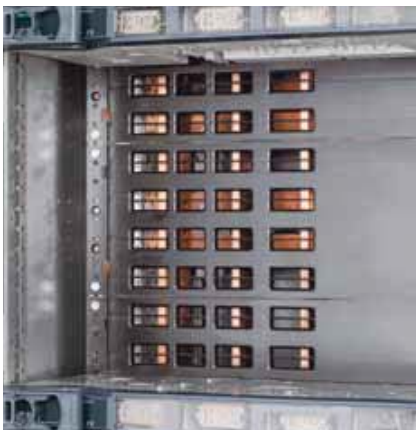
Plug-in busbar system, with test finger safety cover (IP20B).
